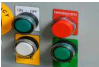
Control panel labels
