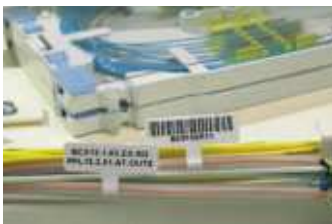
Fibre optic cable markers
