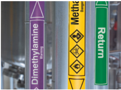
Pipe & valve marking
