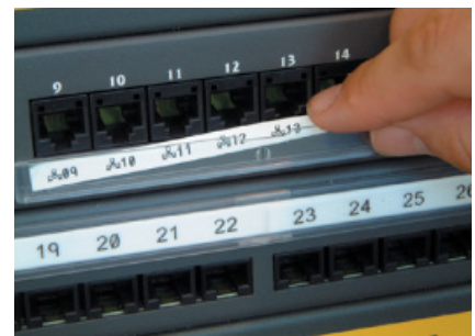
Punch block & patch panel labels
